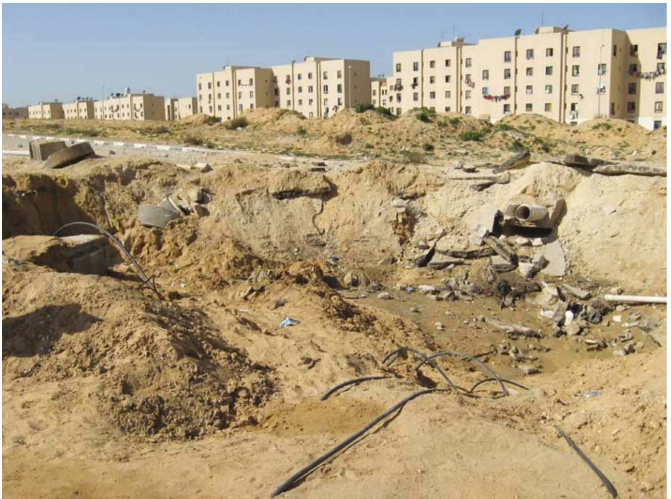
PH1 Crater water pipe damaged. Photo by RS during site visit.
